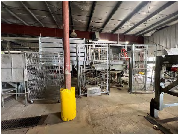
Controlled Atmosphere Stun Area
