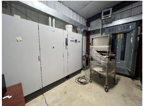
MCC of Live Hold Shed
